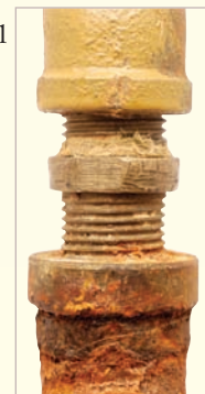
Corroded iron pipe.
