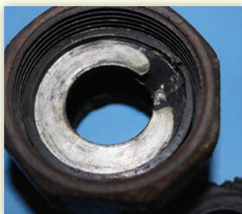
Above: Arcing damage inside black steel fitting melted steel visible upper right.
